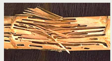
Figure 6. Damage caused by carpenter ants. Note smooth tunnels and lack of sawdust or frass.
